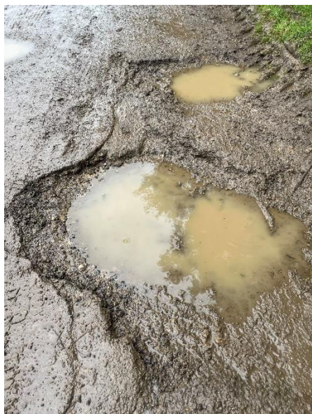
Potholes, rural Oxfordshire
